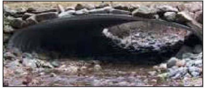
Photo (above): Fish Passage Culvert which is fish friendly
